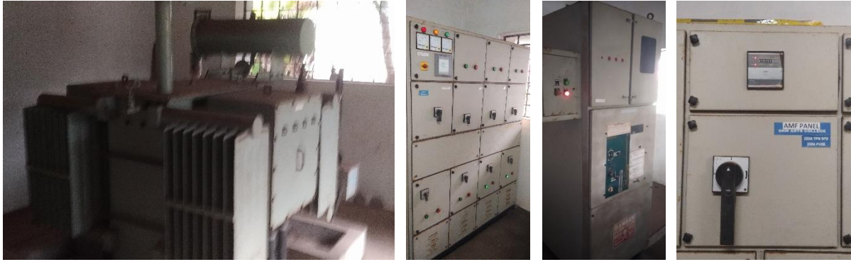
Figure 2.2: (a): Transformer, (b): Main Panel, (c): APFC Panel, (d): SNM College Feeder
