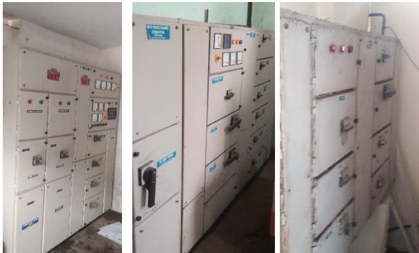
Figure 2.2: (e): AMF Panel (Main Panel- SNM College), (f): SSB 1, (g): SSB 1A
